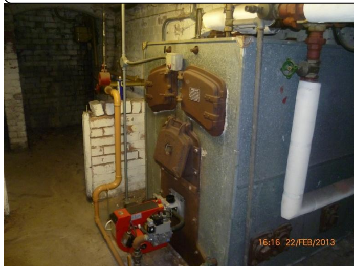
Fig. 4. Gas boilers converted from burning coal
